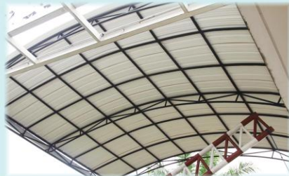
Rangka baja hollow conventional + penutup atap spandek uPVC.
